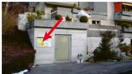
Bürgstrasse Nr. 23, an BKW Trafostation
